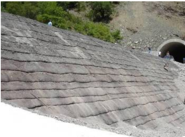
Figure 7. View of the final geometry of the reinforced embankment along a section of the Arta – Trikala highway (see also Figure 1).
