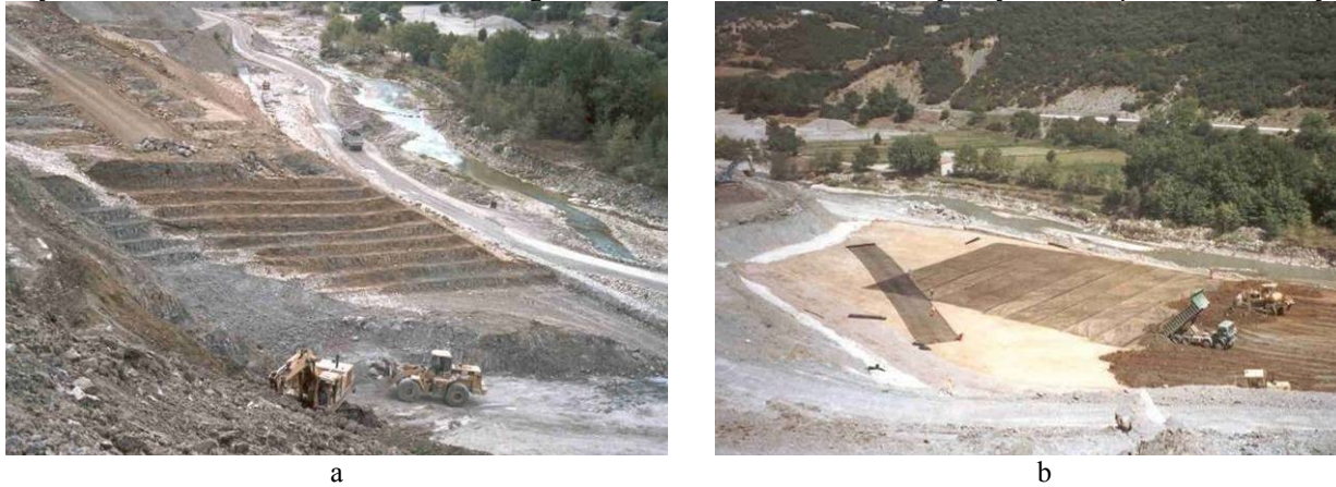
Figure 4. Photographs taken during reinforced embankment construction along the Egnatia highway (see also Figure 2). a) Foundation excavations for the embankment anchoring - b) placement of geogrids and backfilling process.
