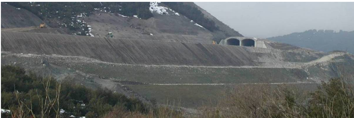
Figure 5. View of the final geometry of the reinforced embankment (see also Figure 2). Commencement of vegetation growth.
