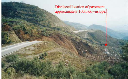
Figure 1. View of disrupted highway section due to landslide.
